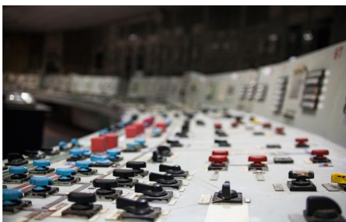
Figure 10-3. Nuclear power plant control panel
